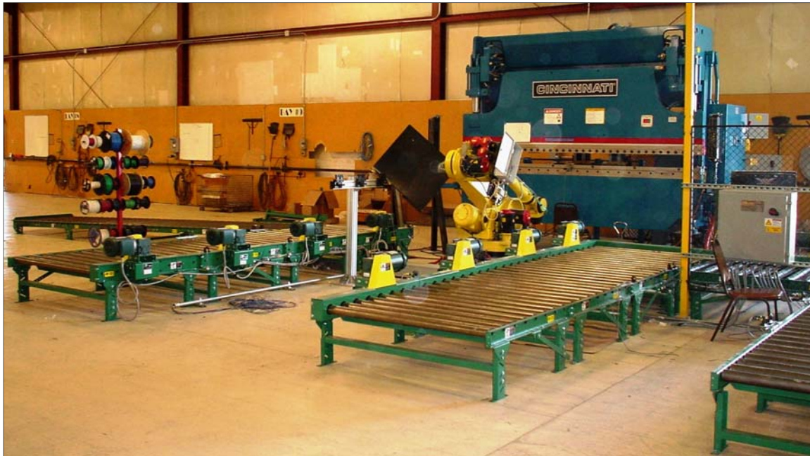
A typical RIBS system with inbound / outbound conveyors, re-grip stand and Robot tool storage station.
